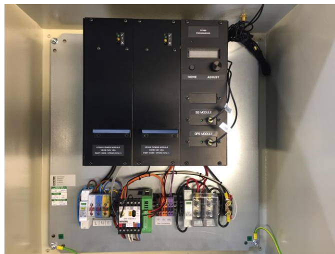
PARALLEL CP500 INSTALLATION – 50V 20A
